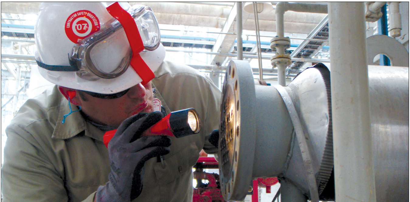
Non-destructive testing (NDT) inspector examines new pipe to ensure safety and quality.
